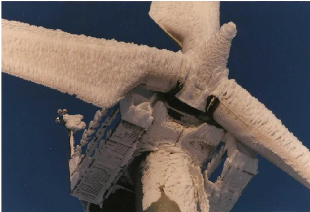
Photograph 3: turbine heavily iced, did not run through icing period
