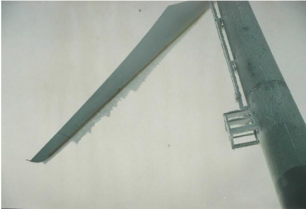
Photograph 5: wedge shape build up from back, note clear back of blade – leading edge heaters not working
